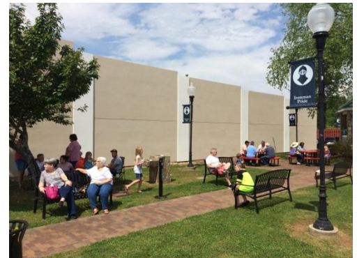
THE REPAIRED WALL, REPAVED PARKING AREA, NEW OUTDOOR FURNITURE, PLANTERS AND ICON BANNERS ADD TO THE MINI-PARK’S WELCOMING AESTHETICS AND UTILITY
